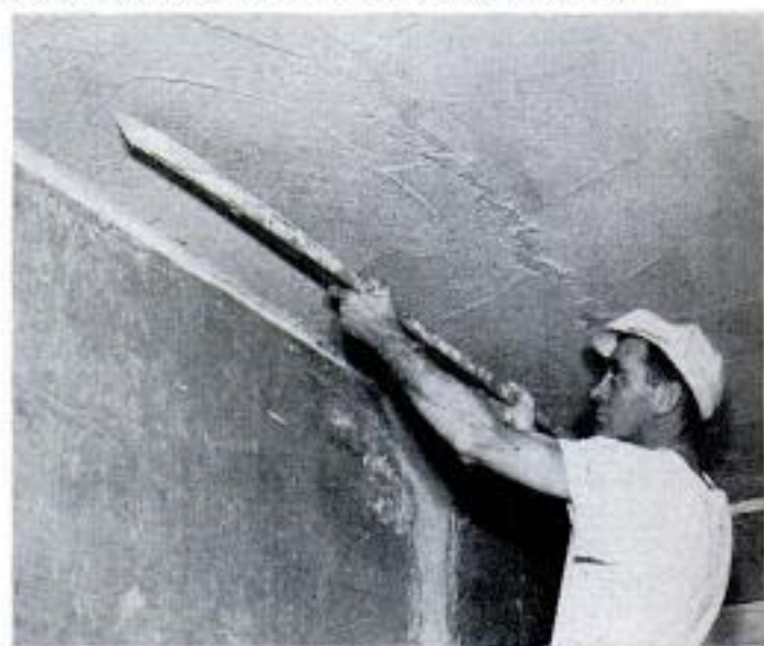
Plasterer uses rod (straightedge) to level surface and remove excess. Final leveling is done with darby (long float) which also produces roughened surface
